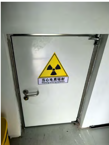
PET/CT机房和高活室之间落地传递窗 (6mmPb)
